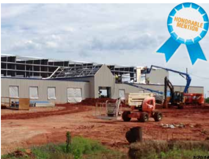
Photo: Courtesy of Alan Lange The Alabama Aircraft Support LLC in Enterprise, Ala., is a 65,000-square-foot hanger equipped with the latest technology to provide maintenance, repair and overhaul services for civilian and military helicopters.
